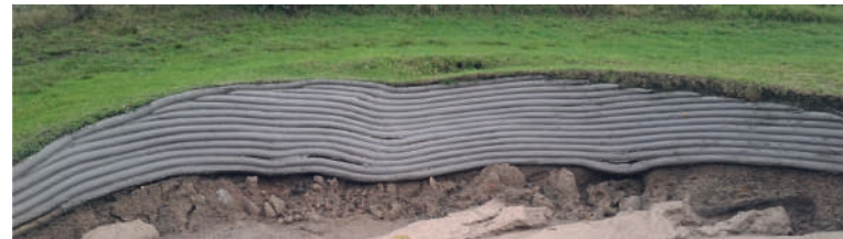
Extensive remedial work was carried out where a bunker wall had collapsed during the storms.
